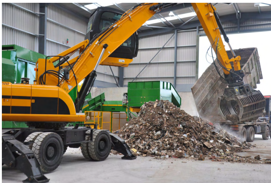
Interserve Material Recycling Facility, Brickyard Road, Aldridge (Reproduced with kind permission of Interserve Construction Limited)
